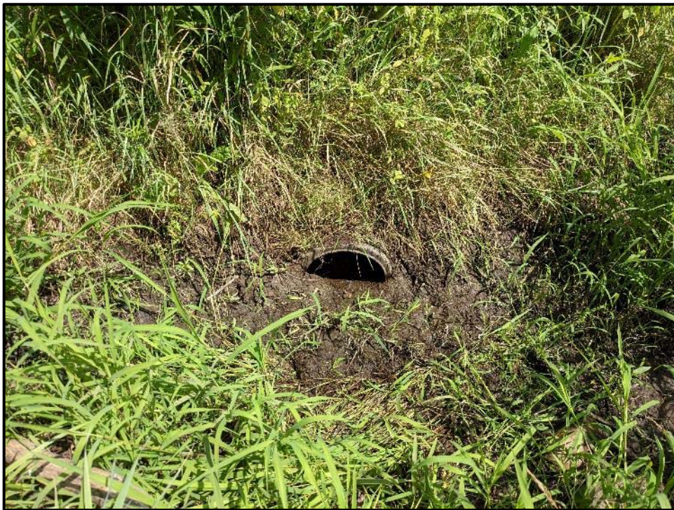
PHOTOGRAPH NO.: 10 FROM: Immediately upstream of farm lane crossing. LOOKING: At small pipe (~300) that conveys flows through crossing.
