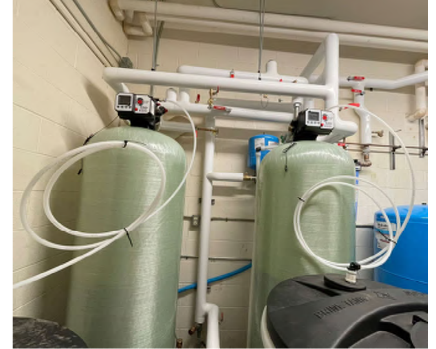
Figure 9 Closer Look at the Water Softener
